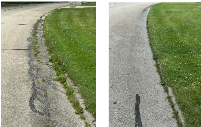
Curbs and gutters which need maintenance
